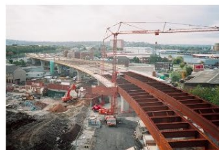
Hunslet Viaduct under construction. De Richard Kay en geograph. Licencia CC BY-SA.
