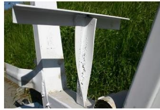
Intentionally twisted (by 90°) steel (equal angle steel) showing permanent deformation. De Sunapeanzler en Wikimedia Commons. Licencia CC-BY-SA.
