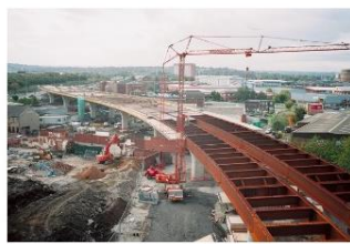
Hunslet Viaduct under construction. De Richard Kay en geograph. Licencia CC BY-SA.
